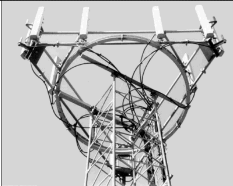
BT Cellnet base station antennae
